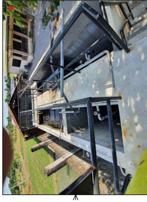
EXISTING STP- OPTION TO REUSE AS CONTROL ROOM OR DISMANTLE & USE THE AREA
