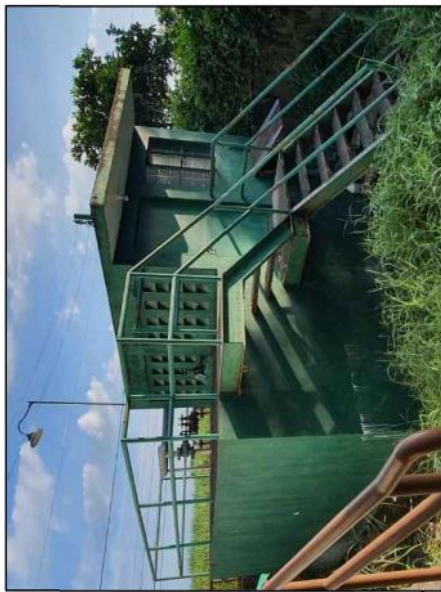
EXISTING STP- OPTION TO REUSE AS CONTROL ROOM OR DISMANTLE & USE THE AREA
